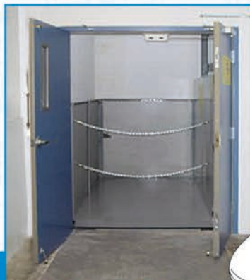
Enclosed Shaftway (Fire Rated)
